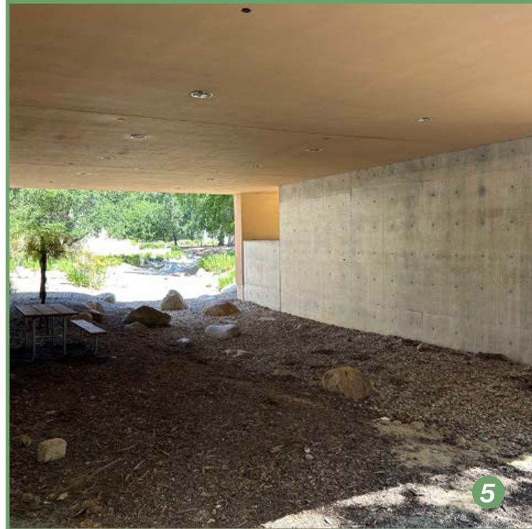
Backside tunnel — underlit passage that interrupts flow and feels uninviting.
