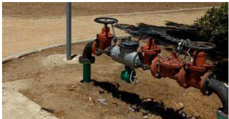
Water valve on site
