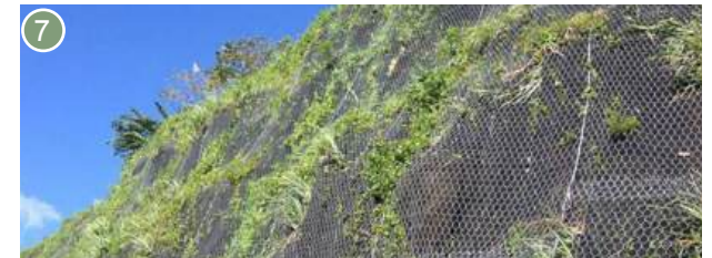
Rock slide prevention netting
