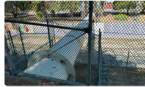
Above Ground Pipe
