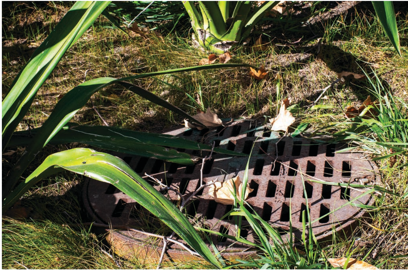
Not a sewer. A dry well!
