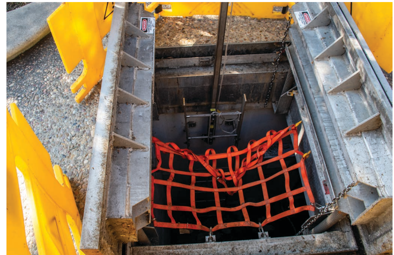
... super secret hidden Fountain Pump Service Room concealed under your feet.
