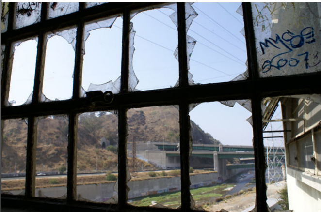
Vandalized interior of the Lincoln Heights Jail. Photo by Danielle D.1
