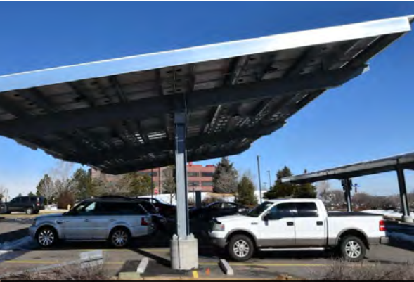
SOLAR PANEL SHADE STRUCTURES
