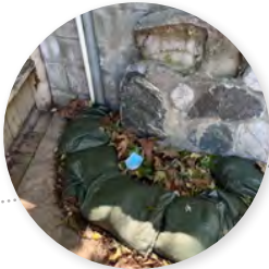
STORMWATER ENTERS ONTO ENCANTO BUILDING SITE
