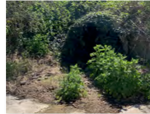
(E) CULVERTED STREAM NEEDS STORMWATER MANAGEMENT'
