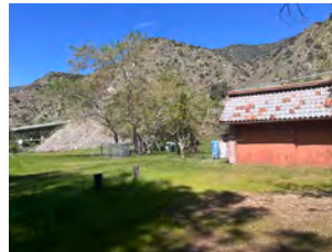
(J) TAYLOR HOUSE AREA HAS DILAPIDATED STRUCTURES
