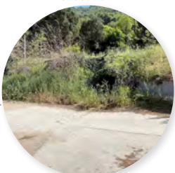
CULVERT FLOW WASHES ACROSS ROAD 2
