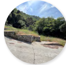
FORMER RV PAD AREA IS STEEP TO VERY STEEP 2
