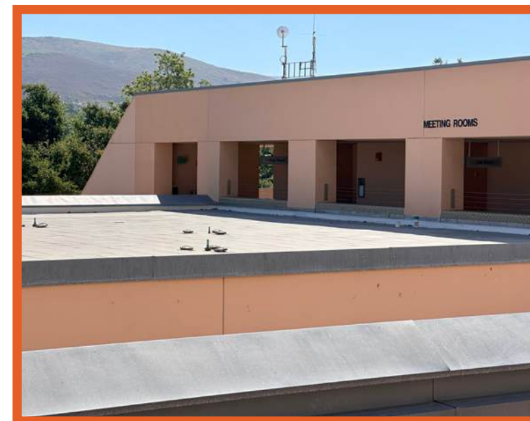
6 Rooftop reflection pool; out of commission due to water conservation concerns.
