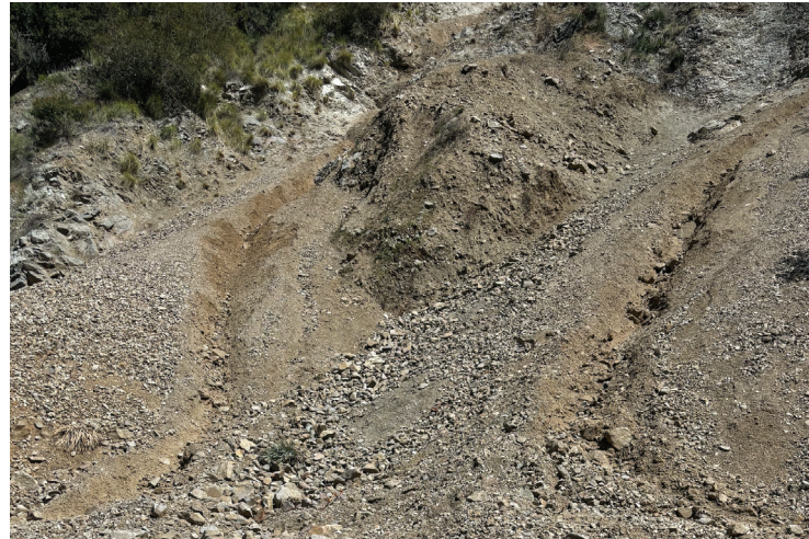
Hazardous landslide area along service road northbound towards dam
