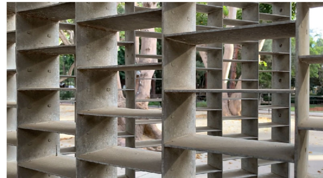
CLOSEUP OF THE ALUMINUM SKRIM FROM INSIDE COURTYARD. THE SKRIM ENCLOSES THE ENTIRE SOUTH WALL OF THE SITE WITH FOUR GATES THAT ALLOW ENTRY/EXIT OF SITE.
