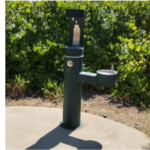
Water Refill Station
