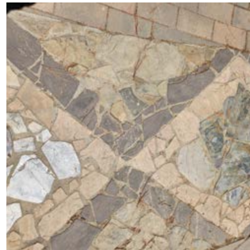
Permeable paving in protected zone paths
