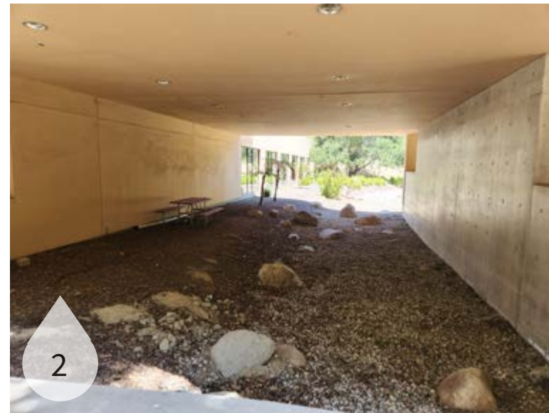
Photo 2: View from path of faux swale that is to close to structure.
