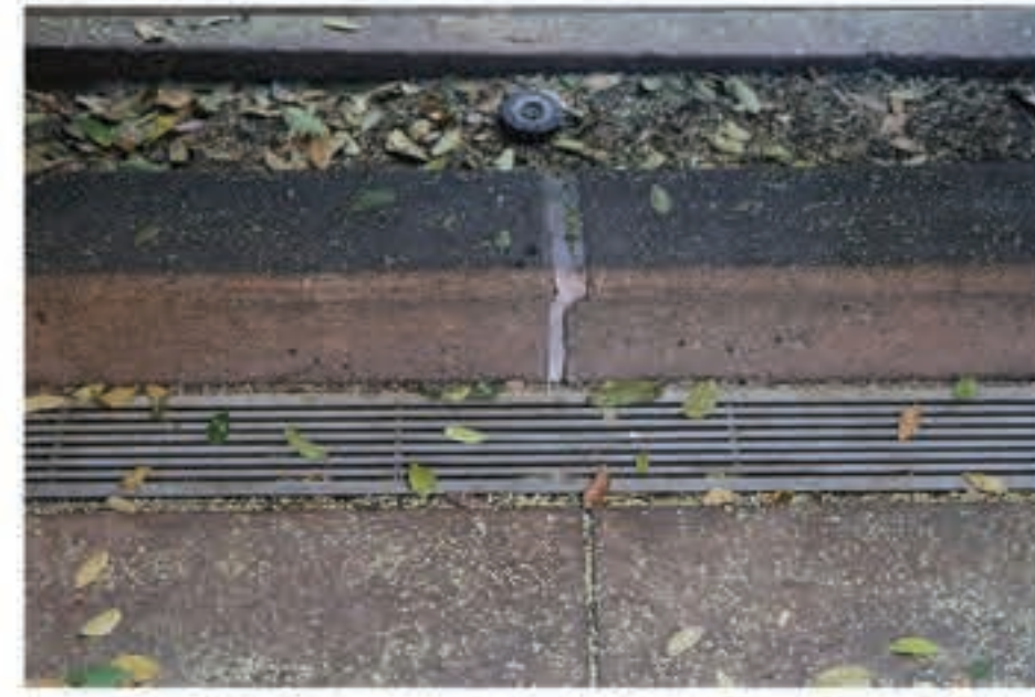
CENTRAL DRAIN WATER LINE/SPRINKLER
