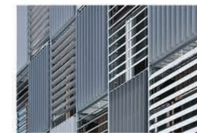
SOLAR LOUVER BRISE SOLEIL TO REDUCE WINDEDDYING AND PROVIDE SUSTAINABLE POWER TO LIGHTS
