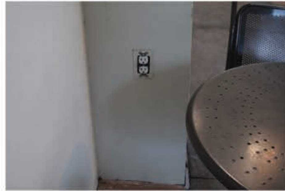
EXPOSED ELECTRICAL OUTLET
