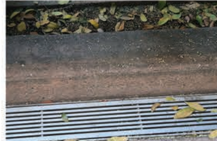
INVERTED DRAINAGE; WASTES WATER AND CAUSE FOUNDATION ISSUES
