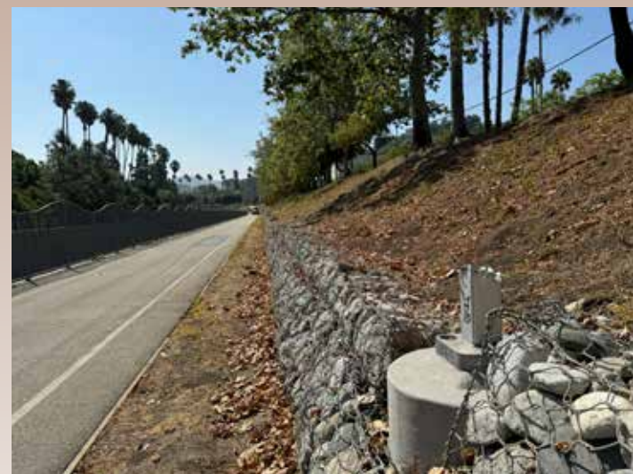
First stripped of their wirings, the street lights are stolen too.
