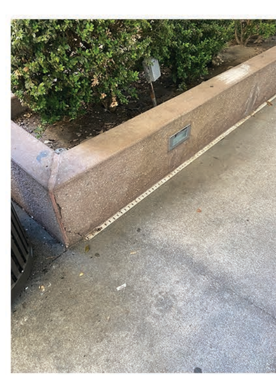
Missed potential of rain water runoff re-use
