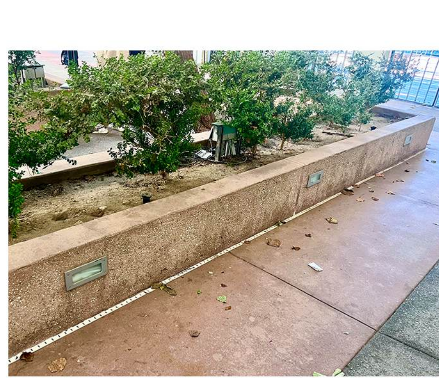
Planter Boxes, Sprinklers, Drainage, Path Lights & Electrical
