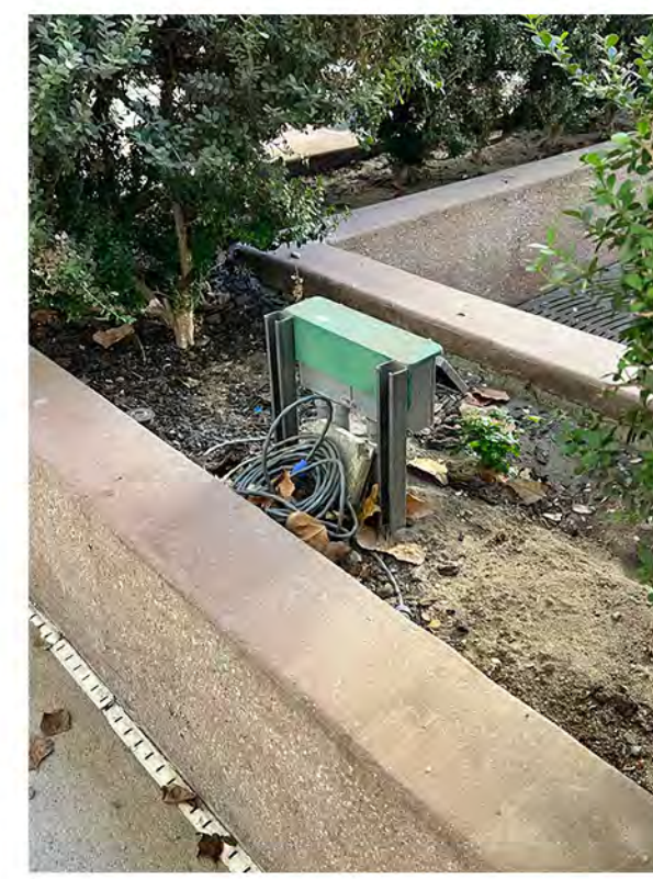
Electrical box with exposed wires.
