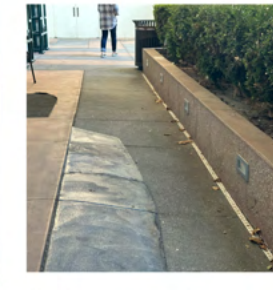
Slight slope shows the possible direction of the water flow towards the drain outlet
