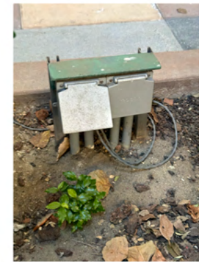
Electrical box situated within a planter bed.
