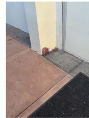
Gas valve located in the NNW wall pillar.
