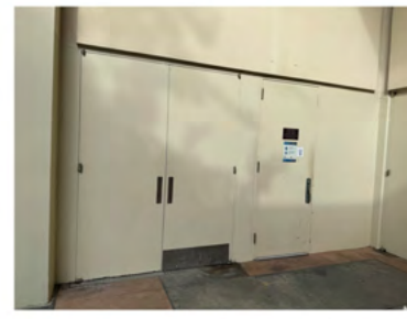
A practical example of the design limitations in one of the corners of the courtyard with multiple doors.
