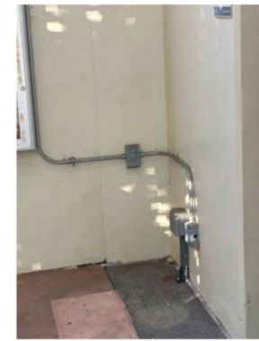
Electrical outlet and Electrical box located in the entrance of The Ralph Freud Playhouse.
