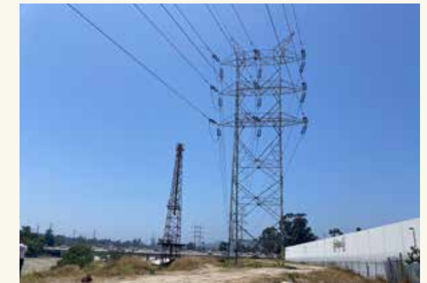
C2 Overhead Power Lines
