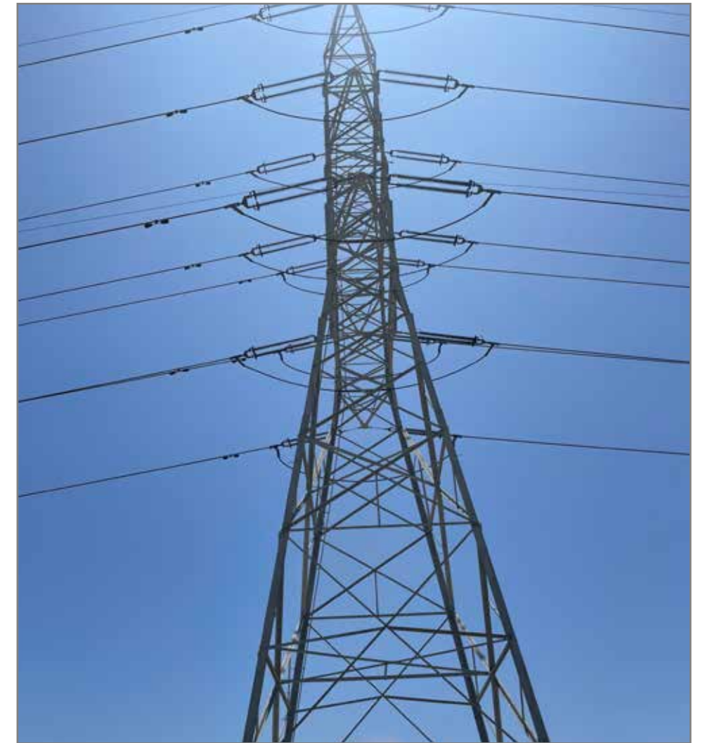
(I) POWER LINE STRUCTURE
