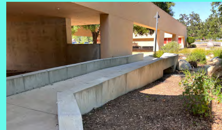
4D Massive concrete paths cut through the existing landscape, making circulation a challenge.
