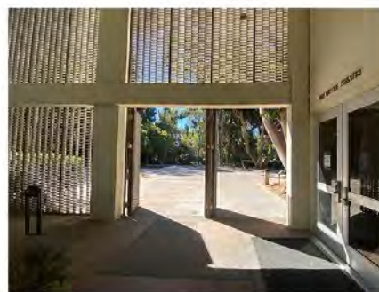
Freud Playhouse and The Little Theater doors open into main entryway, causing traffic congestion
