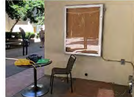
Awkward corner: marquee box + exposed electrical utilities. Currently serving as a seating area, with moveable table + chair.
