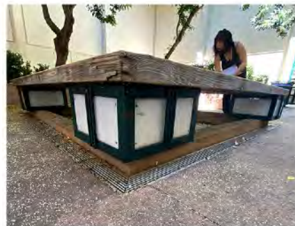
Rainwater flows into one central drain
