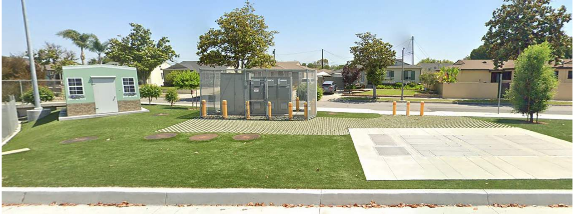
Prefiltration facility (0.2 ac)
