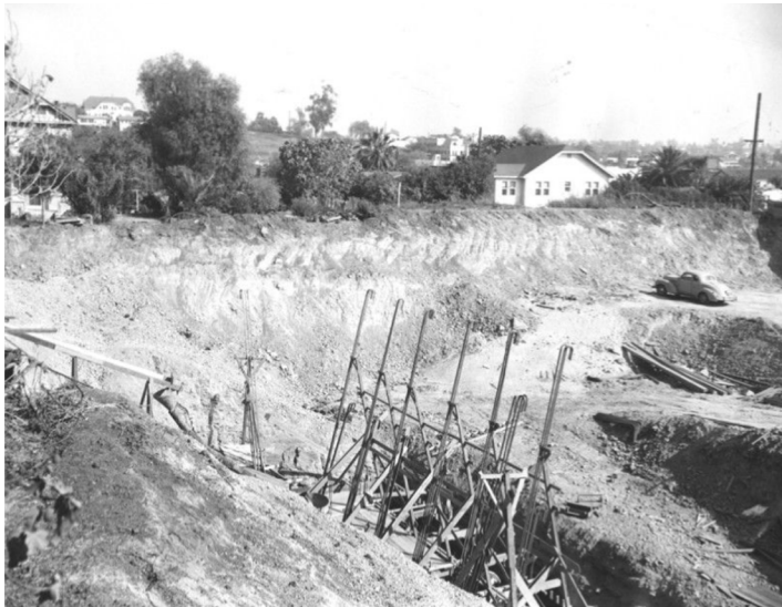
View of Rampart Blvd. and Temple St., where a large "hole" had been dug into the ground for the construction of one unit of the projected Hollywood Freeway, the Benton Way Bridge. Circa 1946.
