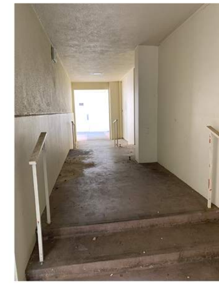
HALLWAY ADDED AT SOMEPOINT DRAINAGE ISSUES LOW CEILING AND NOT INVITING
